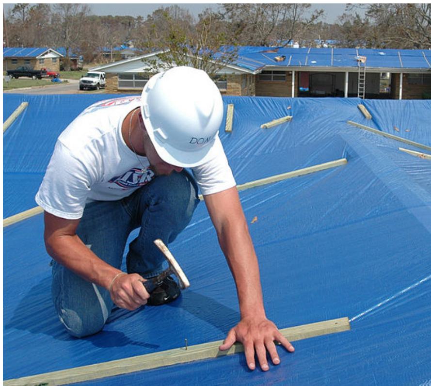
Contractor installs the Blue Roof on Biloxi, Mississippi homes damaged by Hurricane Katrina. Photo by The U.S. National Archives
